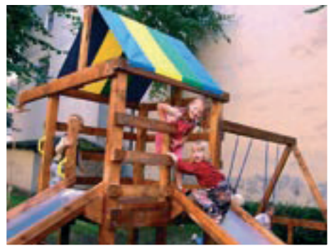
Little did Dave Harless realize when he built this playground that it would begin an ongoing playground construction program embraced by other American and Latvian churches.
